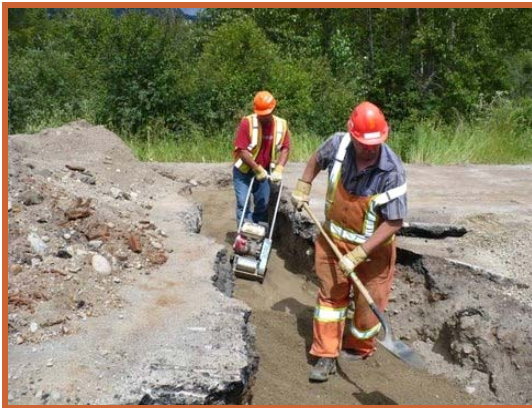
Below — Lynn Davey and John Priede performing sinkhole repair on North Fork Road in July.
