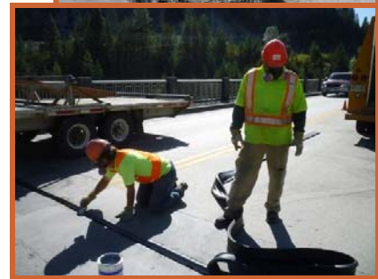
On the right—Ian Stanchuk & Rob Konkin installing a joint seal at Brilliant Bridge near Castlegar.
